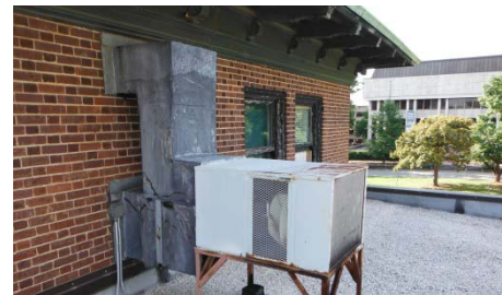
Photo 10. Asbestos-containing black HVAC mastic was found on ductwork insulation located on the roof of the west wing.
