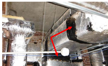
Photo 1. Asbestos-containing black mastic was found on HVAC duct wrap in the east and west wings.
