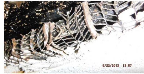
Photo 3. The asbestos-containing plaster ceilings were found above the ceiling grid in rooms 135, 137 and 138 of the east wing.
