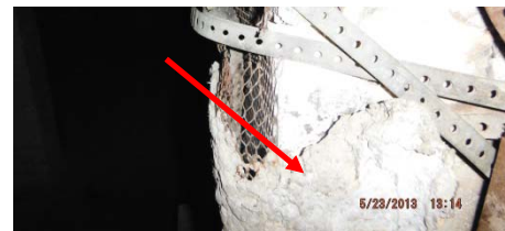
Photo 8. Remnants of asbestos-containing TSI jacketing were found to be severely damaged.
