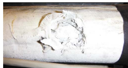
Photo 2. Asbestos-containing Aircell pipe insulation
