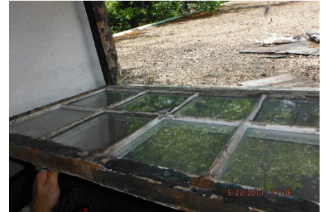
Photo 9. Asbestos-containing exterior window glazing was found on all exterior windows of the subject structure
