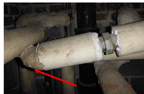
Photo 5. Asbestos-containing mudded elbows were found on pipe lines insulated with Aircell and block insulation.
