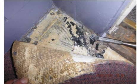
Photo 6. Asbestos-containing 9” x 9” floor tiles were found beneath non-ACM carpeting. Non-ACM felt paper was also identified in this location beneath the ACM floor tiles.
